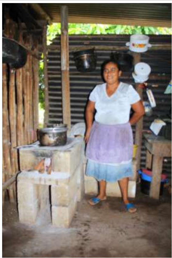
An installed stove. Note that the main body sits on a slab. Wood is pushed in and ashes are removed through the square hole in one end, and smoke leaves to the metal chimney via the round hole in the other end.
